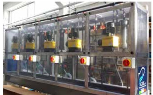
1. Clear Polypropylene Segregation for Dosing Pump.
